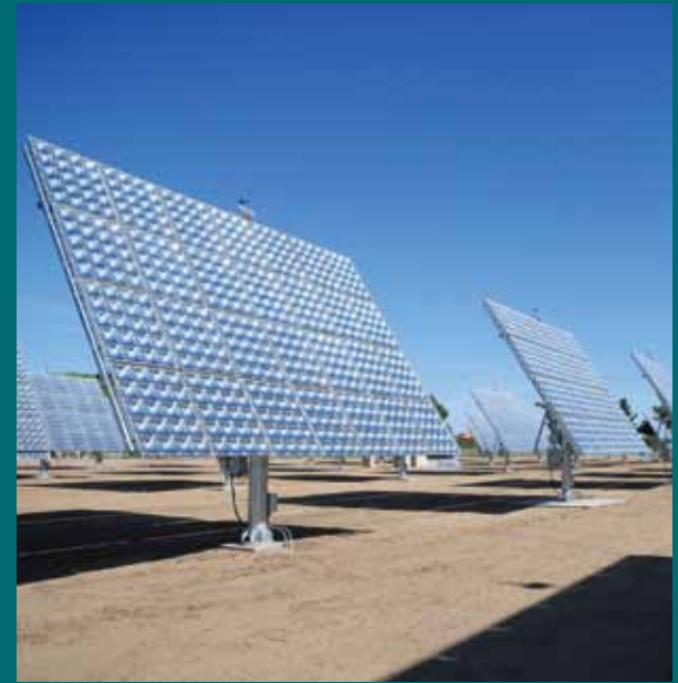
Figure 17: Example of SolFocus CPV Installation
