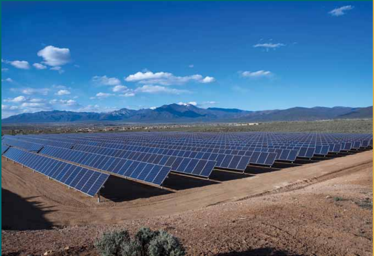
Figure 15: Large Scale PV Plant
