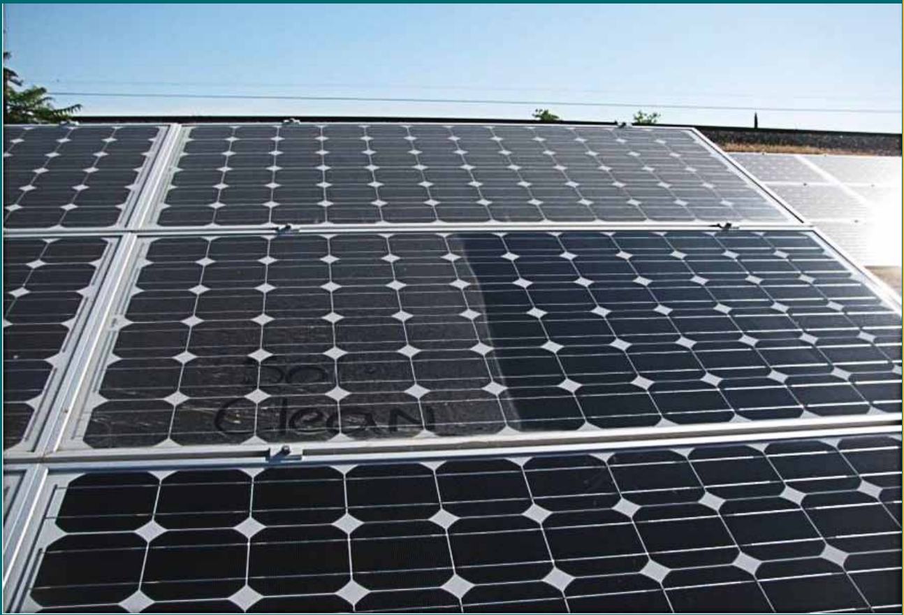
Figure 25: Solar Panel Covered with Dust
