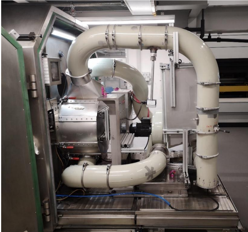
Electro polished enclosure, in the future also the ducts
