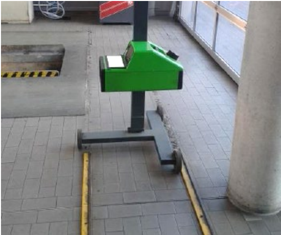
Figure 36: HBS with guide rails which are not being used
