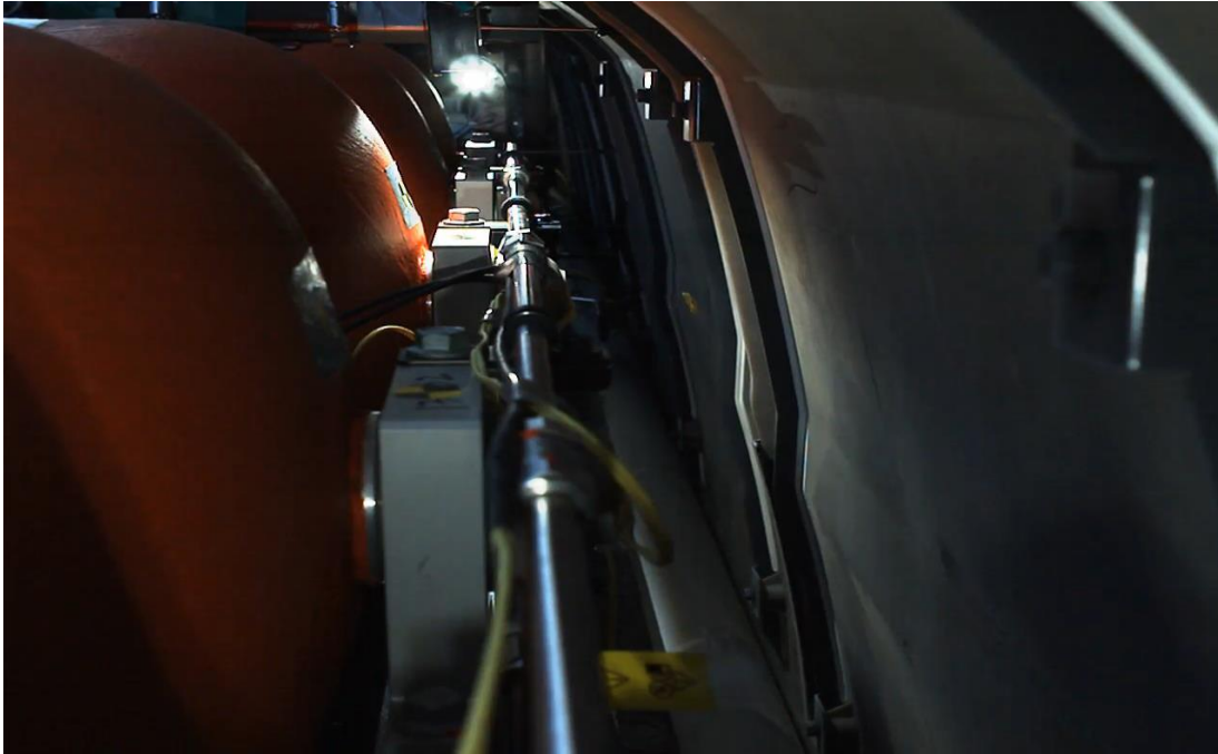
Fuel system (Fuel Tanks and Shut-off valves)
