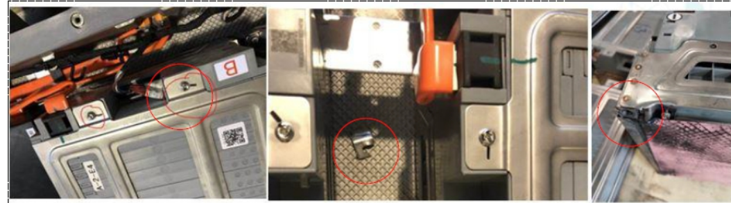
Screw loose, Cracking of conductive metal parts and structural parts
