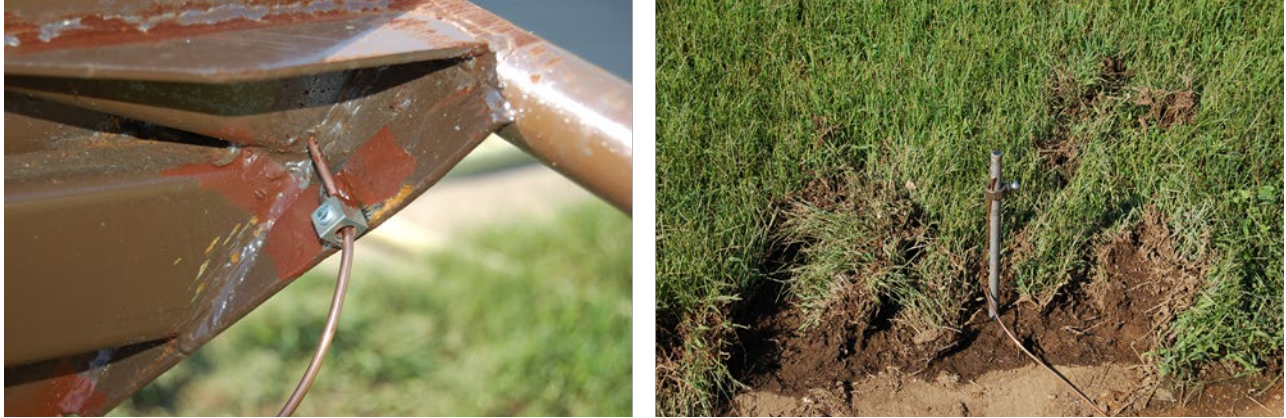
Figure 6. Immersion container grounding connections
