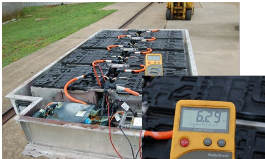
Figure 22. Example confirmation of <50V remaining battery voltage following long-term immersion
