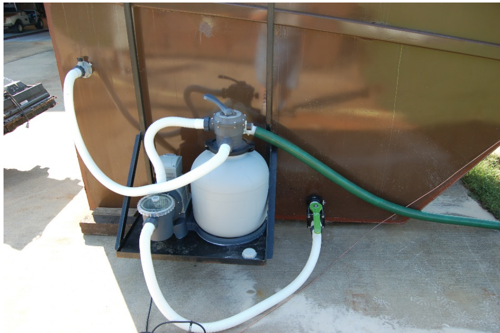
Figure 7. "Pool" filter system for immersion water circulation and filtering
