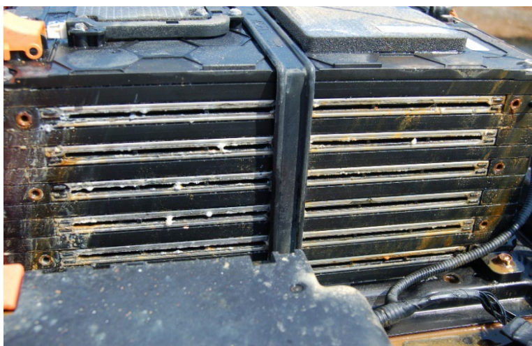
Figure 19. Evidence of battery cell and module degradation
