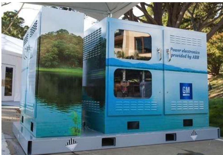
Figure 18 : Microgrid battery backup technology, General Motors, ABB collaboration (Source: gas2.org)
