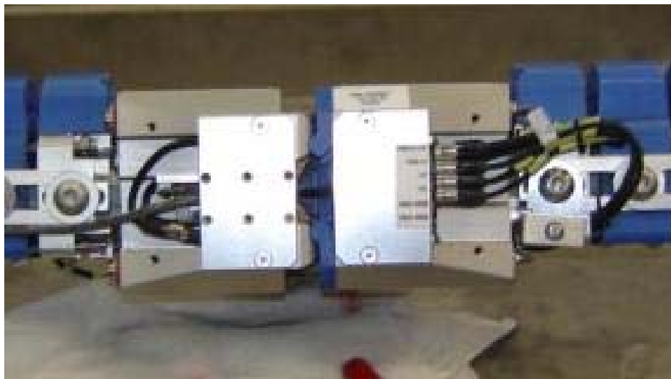
Figure 44 . Right hand side of impact face, lower covers removed
