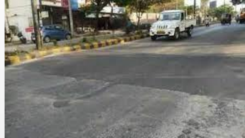
Speed breakers without markings
