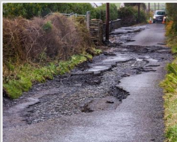
Poor road infrastructure
