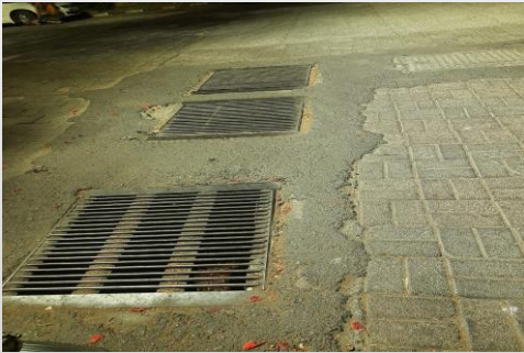
Drainage meshes on road
