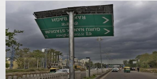
Broken Road Signs
