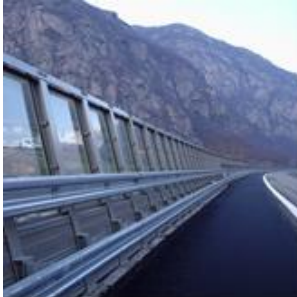
Integrated noise and safety barriers
