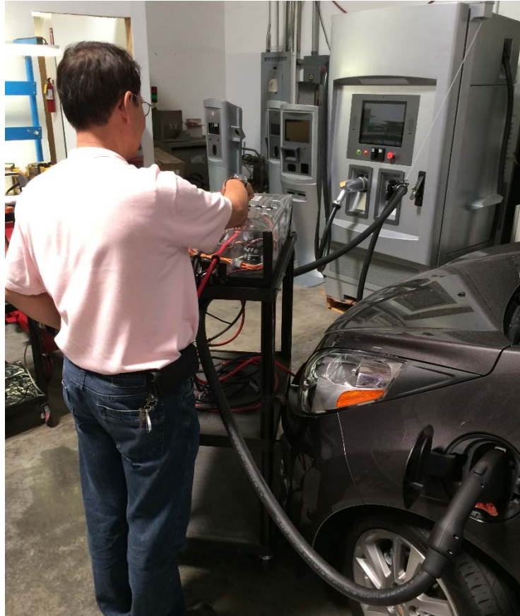
Figure 15 - Engineering charging station with break out box installed.
