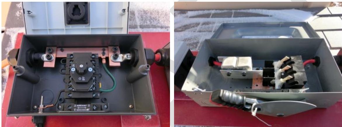
Figure 7 - The interior of a Tap box (left) and the fused short circuit box (right). The fused shorting switch connects directly to the copper bus-bar seen inside the Tap box and to the same component on the other Tap box.
