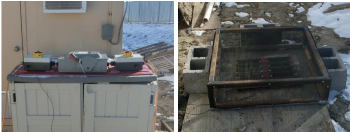
Figure 6 - The switchboard (left) and discharge resistor (right). The discharge resistor is protected beneath a mesh cage to prevent inadvertent contact by an operator. During use a fan provided cooling air across the resistors to maintain their temperature.
