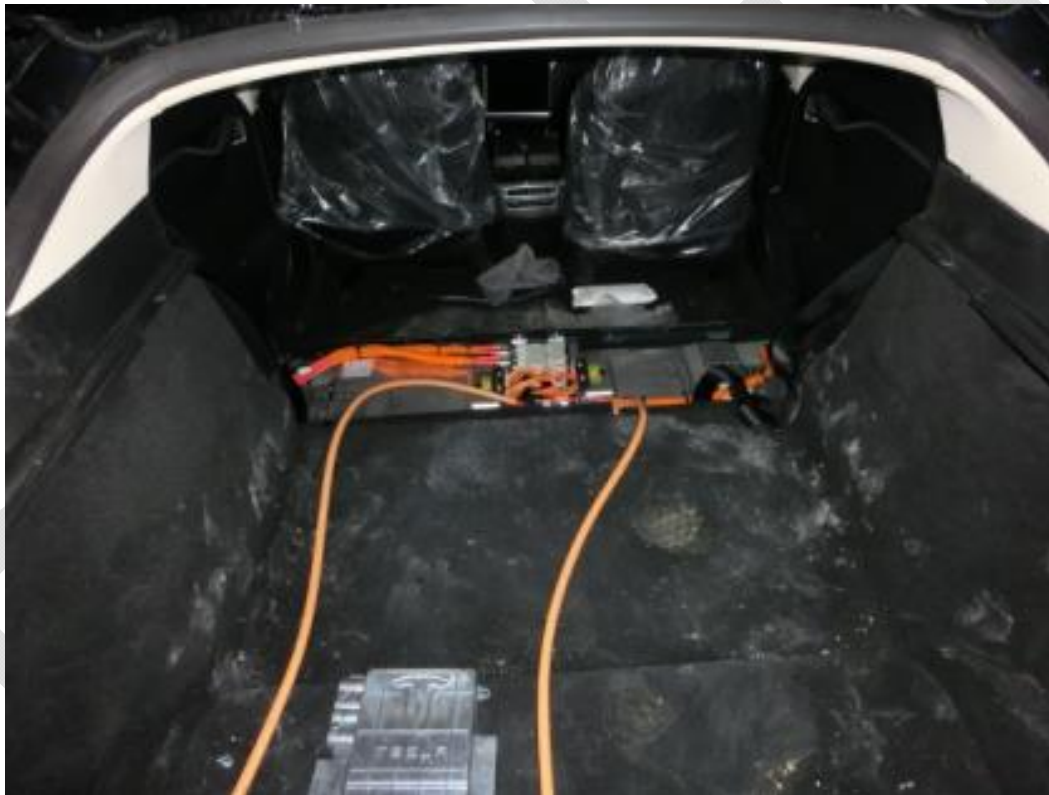
Figure 37 - The location of the exposed DC junction box in the Manufacturer A vehicle. The light orange leads connect to the DC Link. Note that the vehicle rear seats have been removed. The junction box cover can be seen at the lower left of the image.
