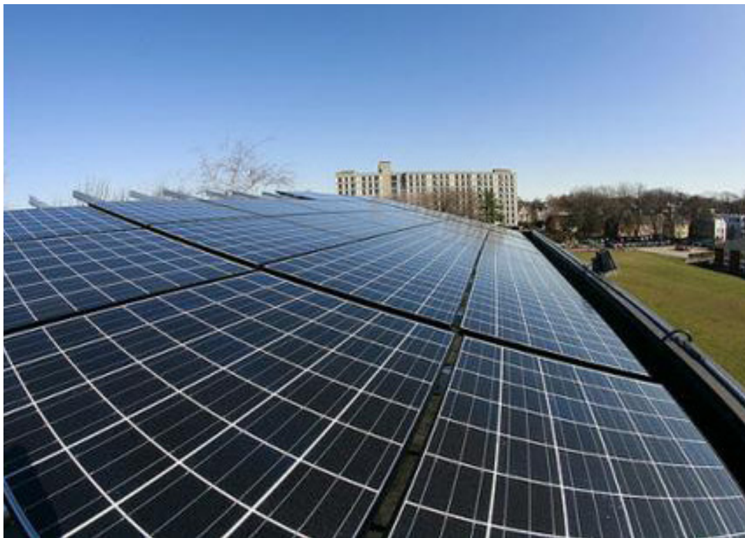
Solar Panel installed in Massachusetts. from: http://power-solar-energy.net/
