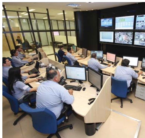
Operational control center, Águas de Guariroba
