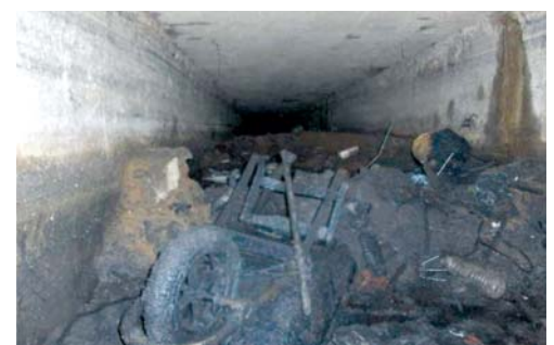
Miscellaneous waste in a sewage collector before cleaning
