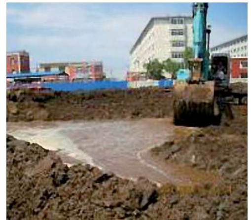
Losses caused by disorderly construction
