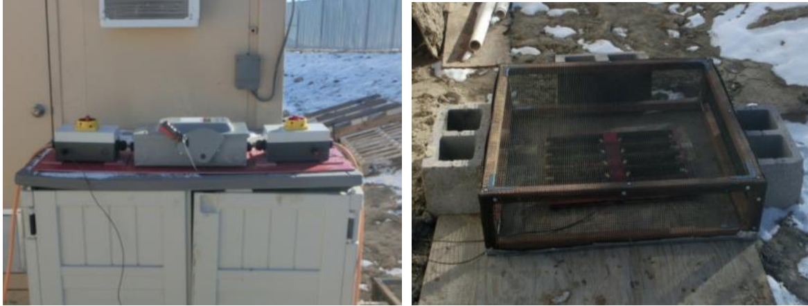
Figure 5: The switchboard (left) and discharge resistor (right). The discharge resistor is protected beneath a mesh cage to prevent inadvertent contact by an operator. During use a fan provided cooling air across the resistors to maintain their temperature.
