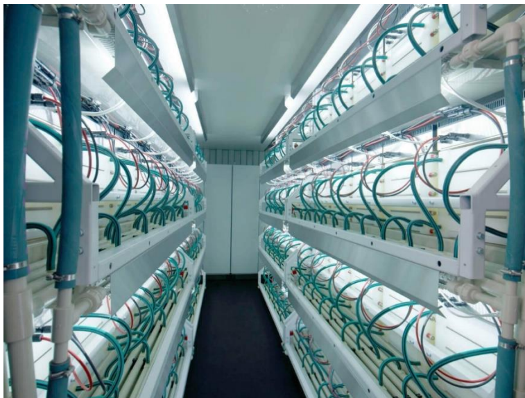
Figure 4.4 Stacks of an all-vanadium system (source: CellCube)
