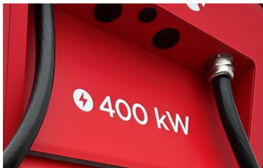
Power rated on charger
