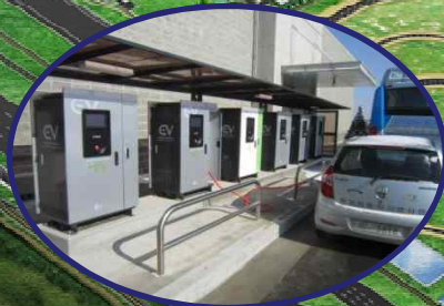
Electric charging station
