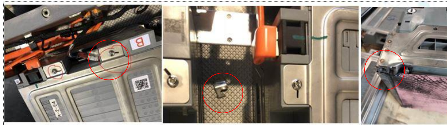
Screw loose, Cracking of conductive metal parts and structural parts
