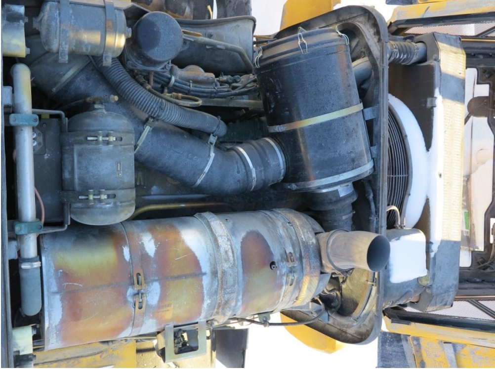
Figure 49 Engine compartment of a wheel loader. Cooling fan is situated in the right part of the picture in a different compartment than the engine.
