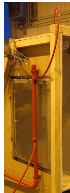
Figure 5. Aspirating smoke detector system.
