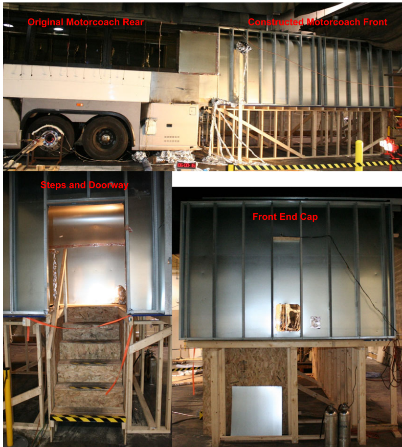
FIGURE 1 Photographs of the motorcoach extension. The top photo shows most of the assembly of the original motorcoach rear half and added front extension. The bottom left photo shows the extension doorway and steps. The bottom right photo shows the front end with the window and visibility camera [Colour figure can be viewed at wileyonlinelibrary.com ]
