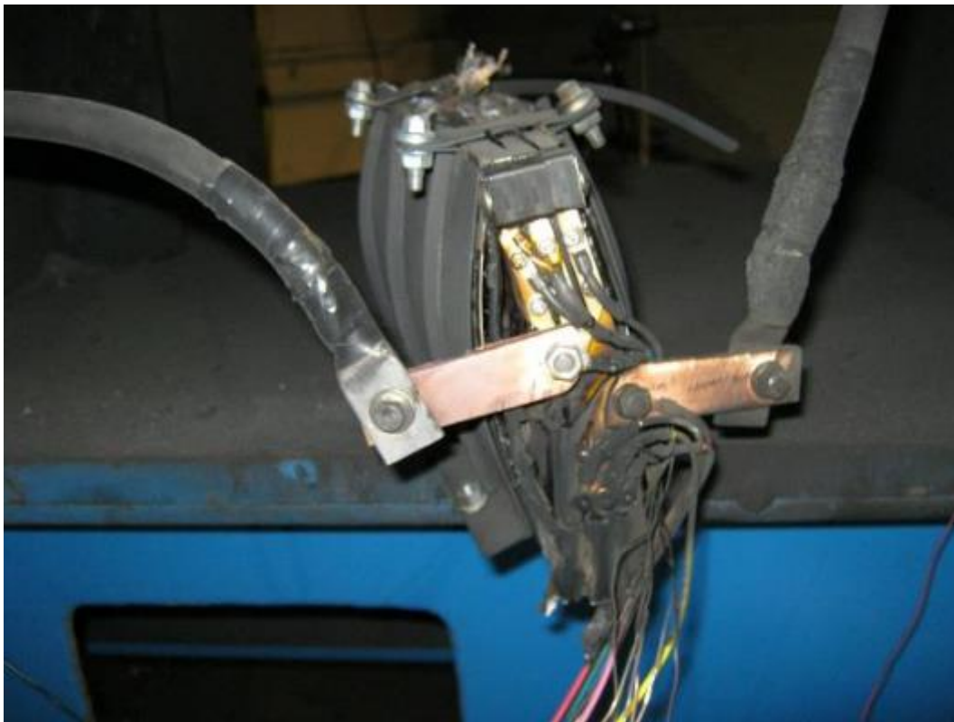
Figure 154 Start/Stop 77A String Type B Post-Test Fixture (OC038)
