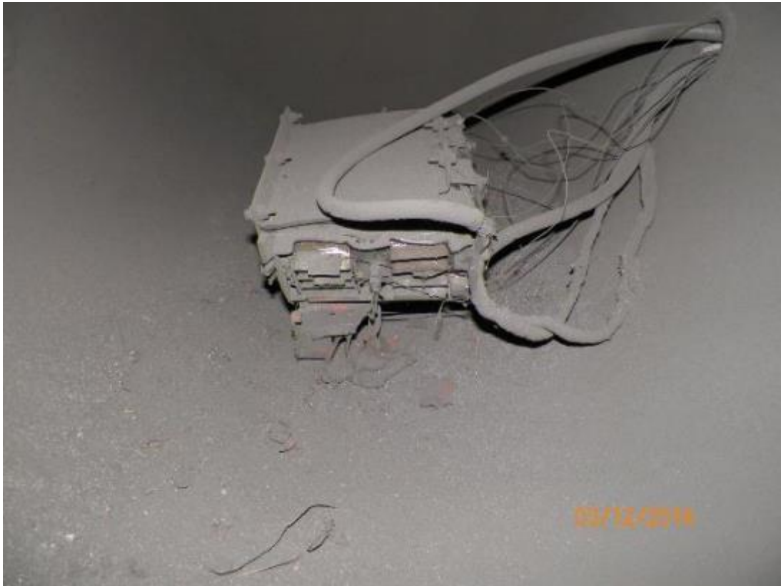
Figure 139 Continuous 155A String Type A Post-Test Fixture (OCPCA02)
