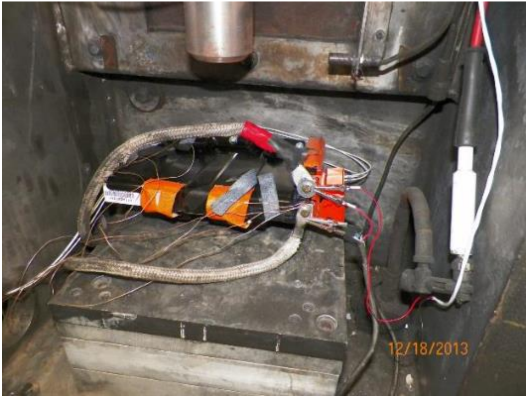
Figure 163 Hard String Type A Pre-Test Fixture (SSHA01)
