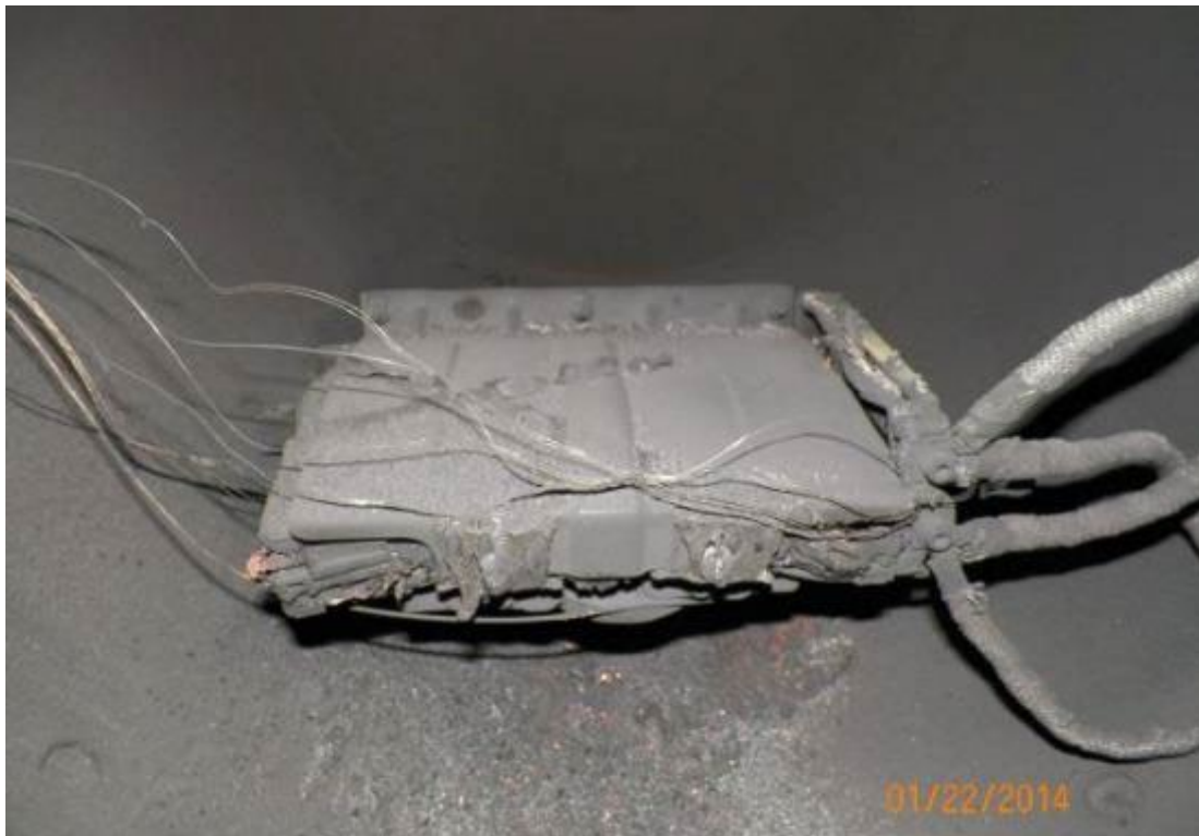
Figure 131 Start/Stop 60A String Type A Post-Test Fixture (OCISA01)
