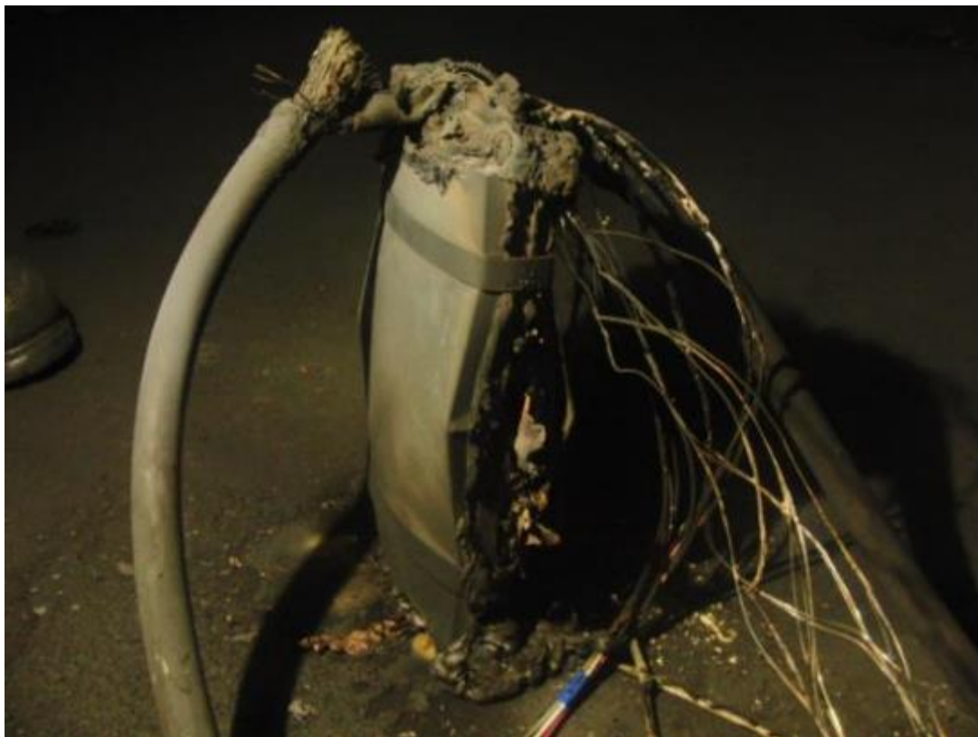
Figure 133 Start/Stop 60A String Type B Post-Test Fixture (OC009)
