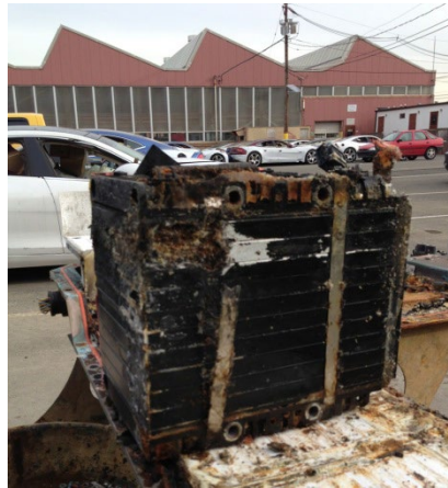
Figure 25: Evidence of actual individual cell damage
