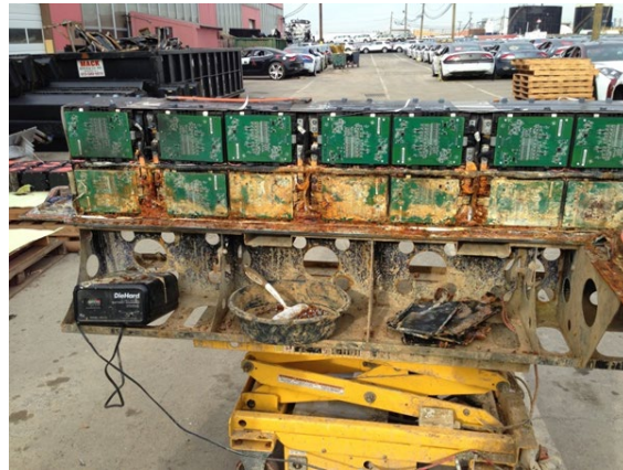
Figure 21: Water Intrusion of the entire pack
