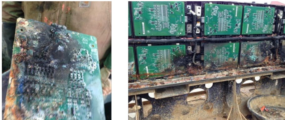
Figure 22: BMS damage and shorting
